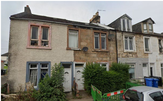
Figure 17 - 1.5 Poor Condition Tenaments
