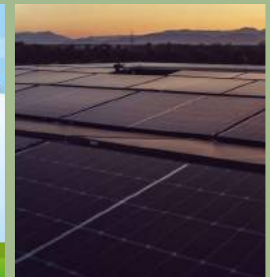
PV panels used for electricity production[43]
