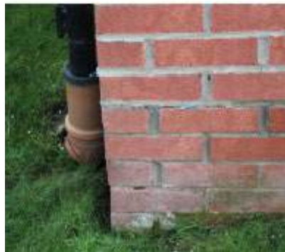
Figure 3 Brickwork not lined up
