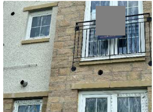
Figure 3 Uneven Windows-Lintel spacings
