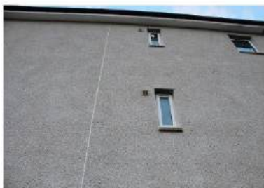
Loose vent cover
