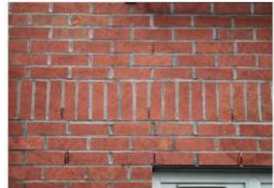
Cavity Vent + Excessive mortar
