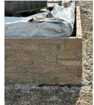
Figure 2 Brickwork not lined up
